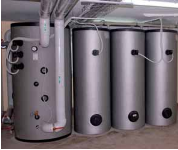
Fot. 1. Bufor TPS800 i zasobniki WWS 507 firmy Alpha-InnoTec (fot. Hildebrant)
